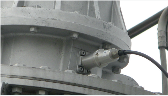
Detail of measurement connection used for bushing diagnostics on the 400 kV side
