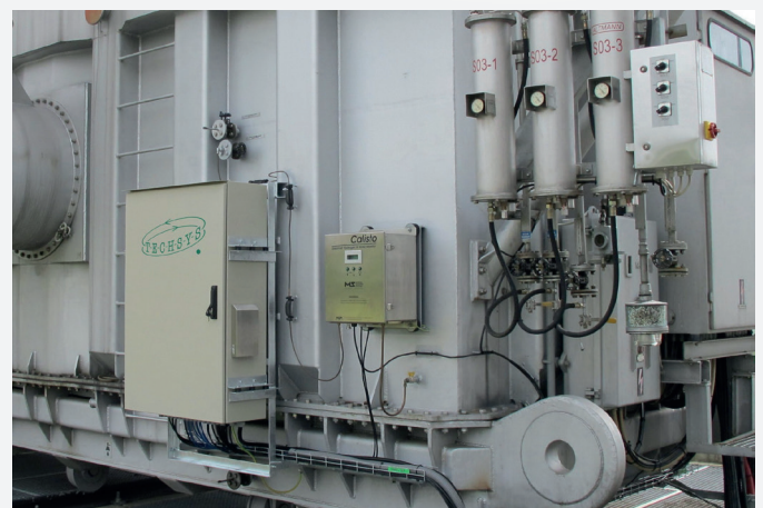
TECHSYS cubicle on the tank of a 350 MVA 400/110 kV transformer
